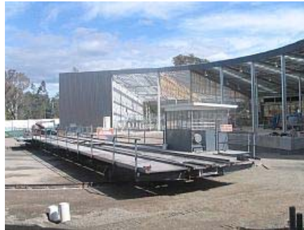
Above: Turntable has been moved from the northern end of the museum site near the new Roundhouse
